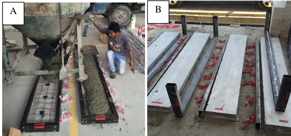
Figure 3: (A) In-situ concrete toppings were poured into each formwork. (B) The concrete slabs and toppings were left dry before being removed from the formworks.
