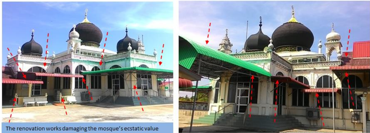
Figure 8: Arrows show the facade defects caused by improper renovation works
