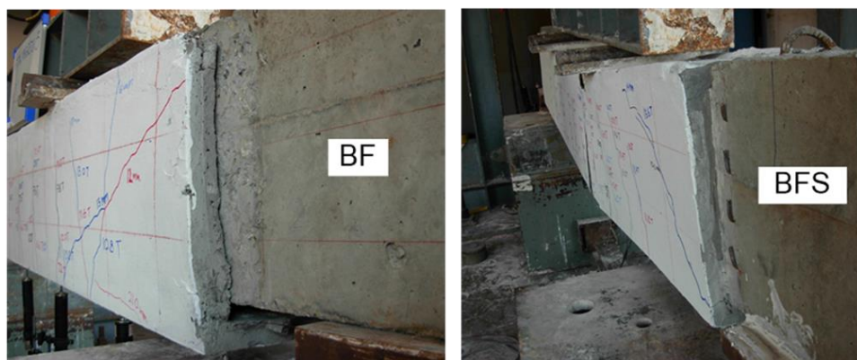
(a) Separation of Ferro-cement from the beam due to the shear flow
