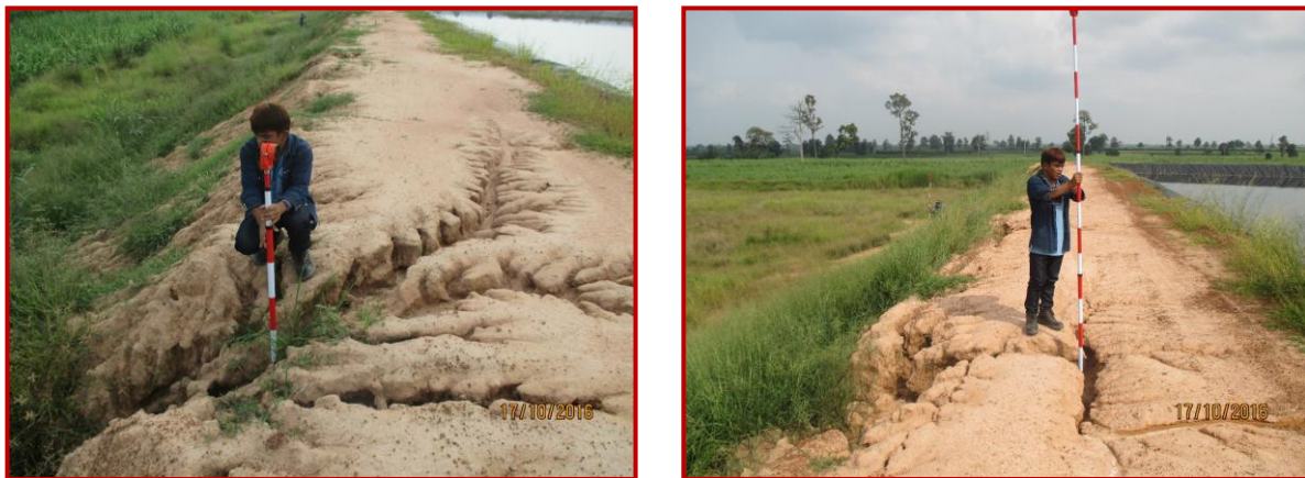
Figure 6: Dispersive soil slope of the Khon Buri Sugar Mill Factory.
