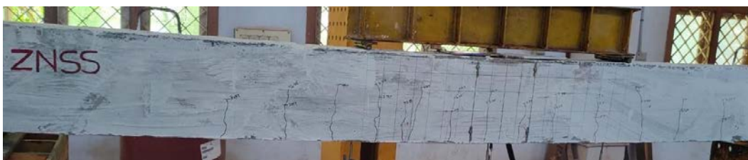
(c) Crack Pattern of ZNSS.
