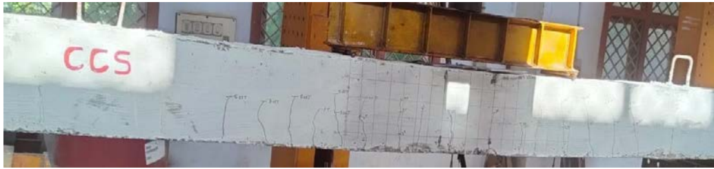
(a) Crack Pattern of CC Beam
