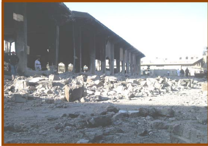
Figure 3: Marketplace, must be rehabilitated and conserve as a social and cultural aspects reflecting the sense of place "Recent issue".
