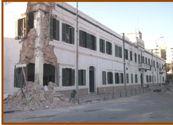
Figure 2: Colonial building damaged during war should be restored and retained “Recent issue.”
