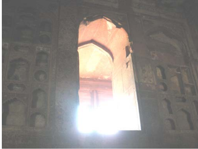
Figure 9: Vent near dome allows hot air to escape.
