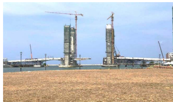
Figure 7: The first drawbridge in Malaysia connecting Kuala Terengganu City Centre to Kuala Nerus (in construction)
