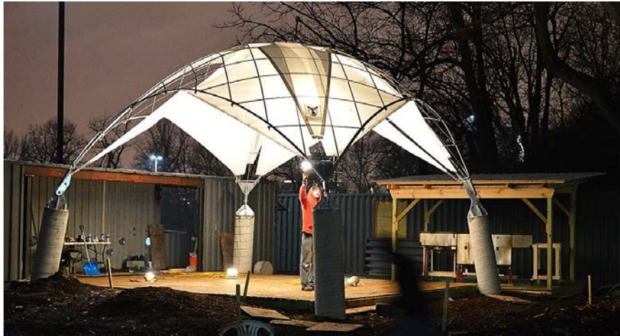
Figure 2: Construction nearing completion on the Gridshell dome at the GRIDfarm, spanning close to 30 feet using only one-inch rebar and clad with a double layer of fabric “sails” made from salvaged material.
